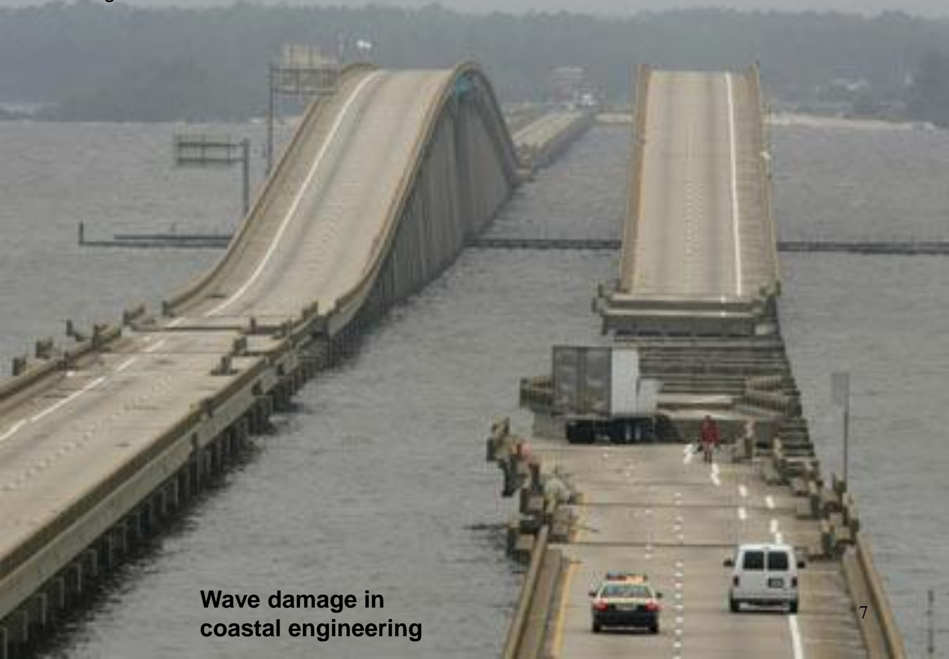
Interstate-10 bridge across Escambia Bay, Florida, after Hurricane Ivan - looking east from Pensacola
